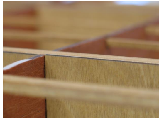
Spar webbing should be flush with rib
